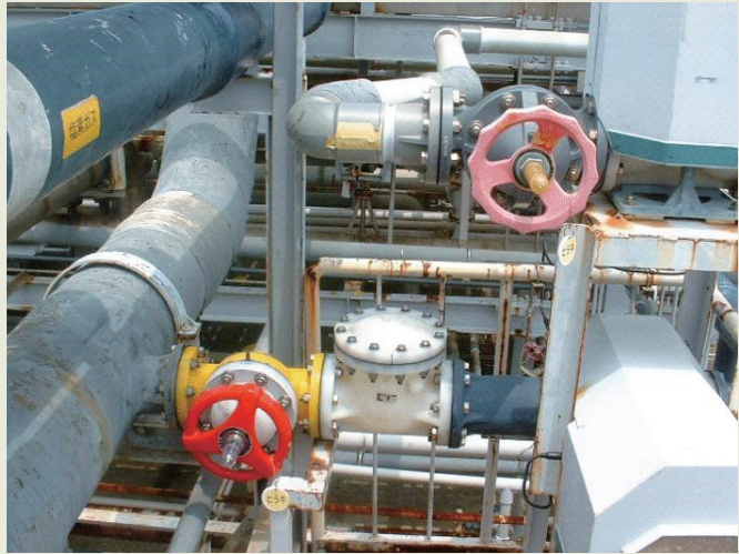
⋈ PVDF swing check valve installed horizontally at a chemical plant and has been working for more than 20 years.
